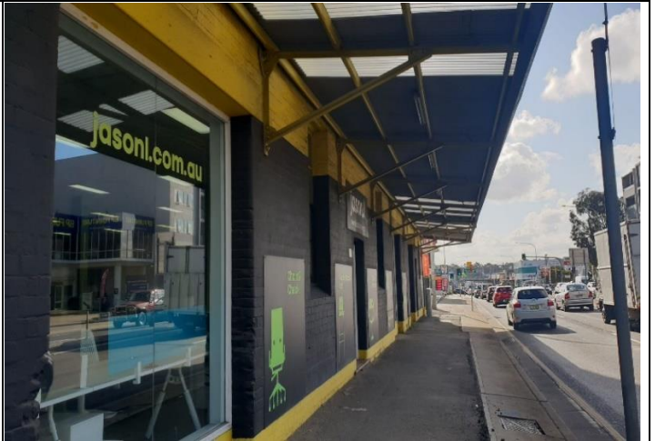
Photo 26: 138 Parramatta Road, metal awning structure, lead containing yellow paint (WSP-064198).
