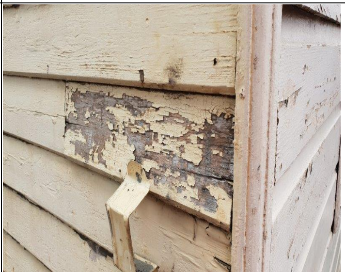
Photo 18: 59 Cowper Street, Dwelling - Exterior, Timber walls surrounding dwelling, lead containing yellow paint (WSP-104432).
