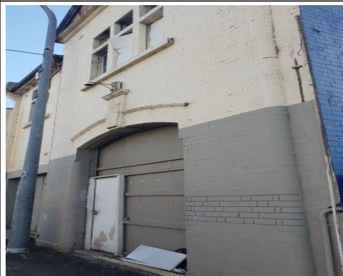
Photo 35: 38 Good Street, eastern Façade brickwork, lead containing white paint (WSP-104459).
