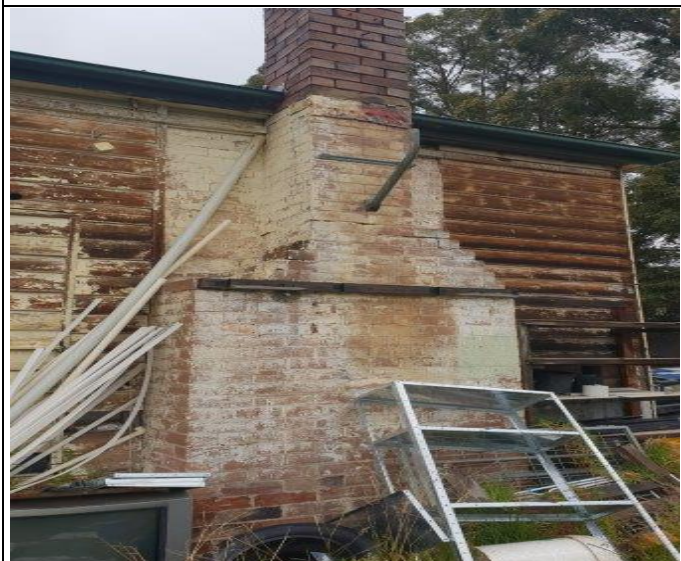
Photo 17: 59 Cowper Street, Dwelling - Exterior, Northern aspect, chimney, lead containing white paint (WSP-104433).
