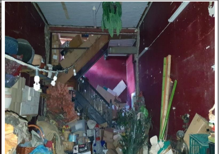
Photo 30: 38 Good Street, ground floor, southern room walls, lead containing maroon paint (WSP-104455).
