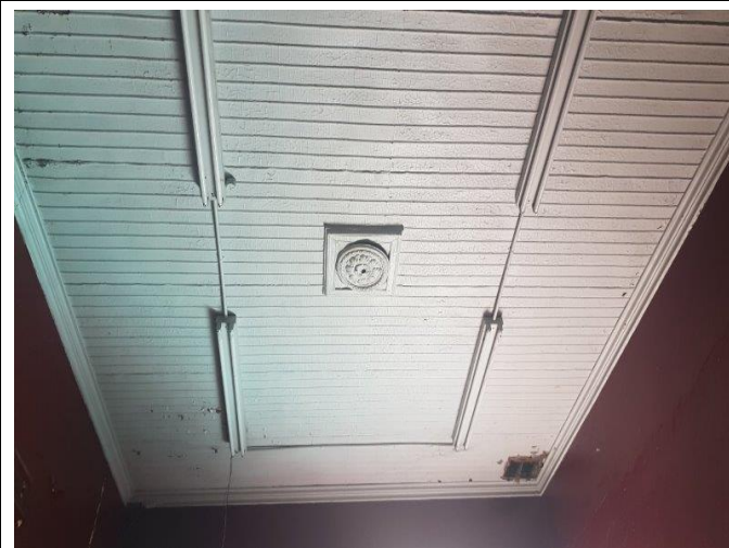
Photo 29: 38 Good Street, ground floor, southern room ceiling, lead containing white paint (WSP-104454).
