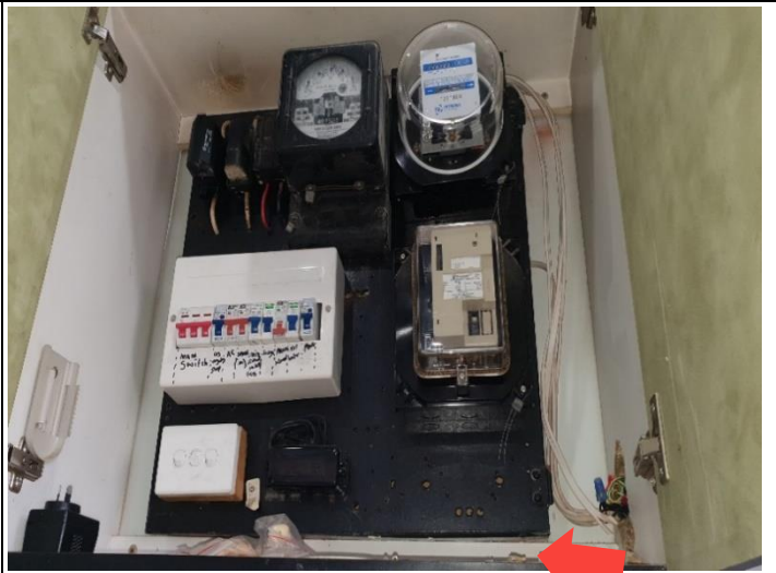
Photo 8: 34 Good Street, northern wall asbestos-containing electrical distribution board.
