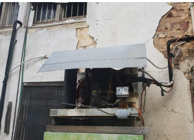
Photo 41: 28-30 Good Street, ground floor, western aspect, adjacent rear carpark, refrigerant, ODS containing material.
