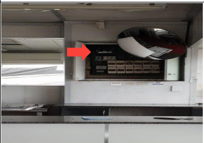
Photo 5: 26 Good Street, northern wall, asbestos-containing electrical distribution board.
