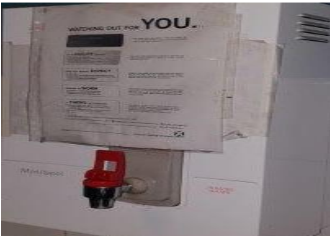
Photo 39: This water heater is the same as identified, 138 Parramatta Road zip brand heater, kitchen
