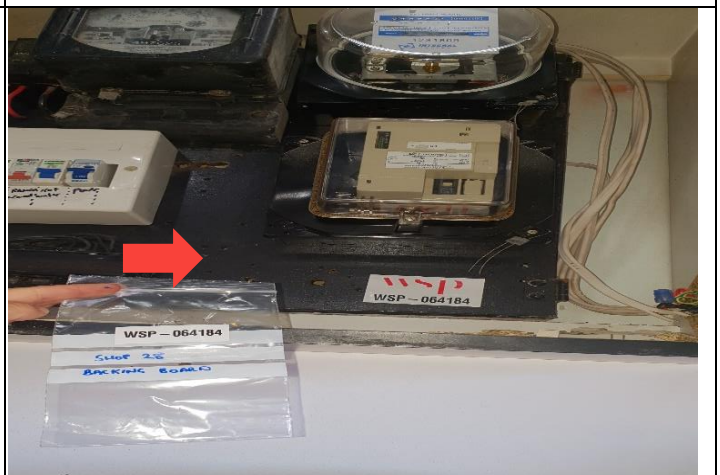
Photo 6: 28-30 Good Street, northern wall, asbestos-containing electrical distribution board.
