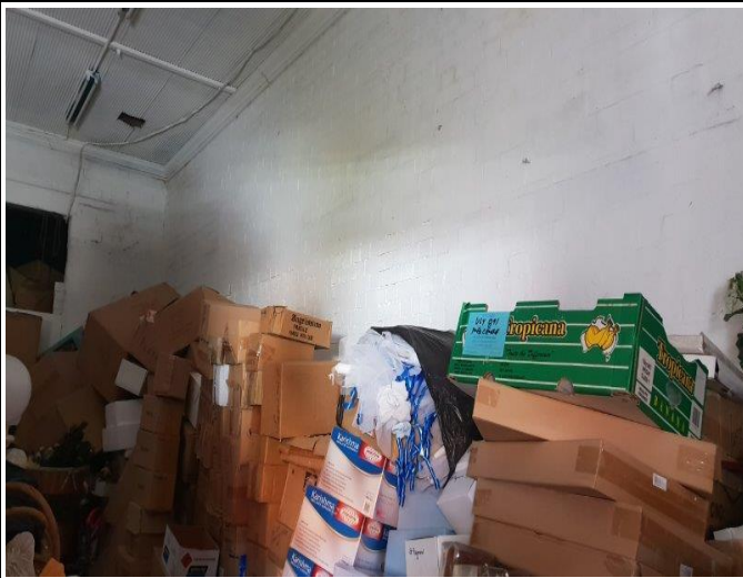
Photo 31: 38 Good Street, ground floor, northern room, walls, lead containing white paint (WSP-104456).
