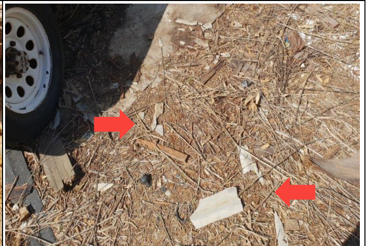
Photo 4: 61 Cowper Street, vacant block, northern aspect to yard, asbestos-containing fibre cement fragments identified on ground surface.
