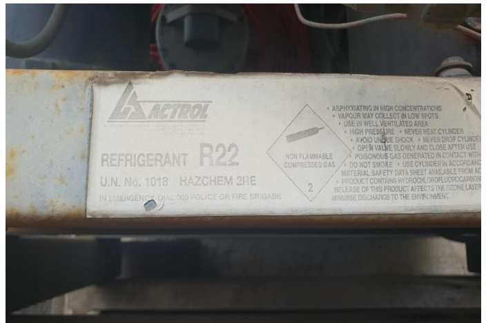
Photo 40: 28-30 Good Street, ground floor, Western aspect, adjacent rear carpark, refrigerant, ODS containing material.
