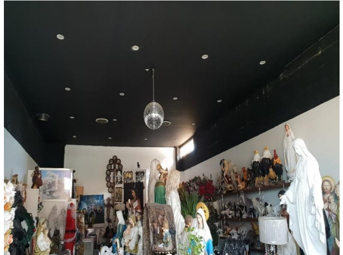
Photo 38: 28-30 Good Street, ground floor, black ceiling tiles contain SMF material.
