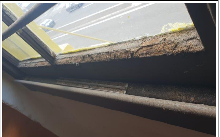
Photo 28: 138 Parramatta Road, window frames, lead containing brown paint (WSP-064190).
