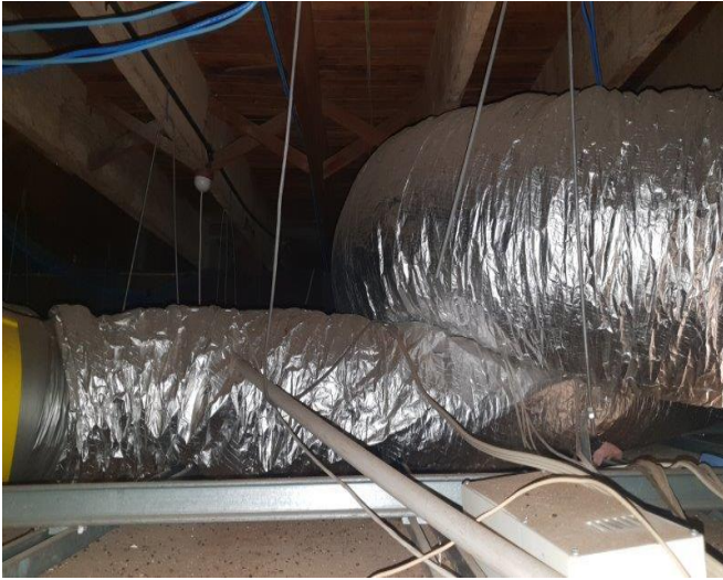
Photo 37: 138 Parramatta Road, ground floor, ceiling space, Flexi-ducting contains SMF.
