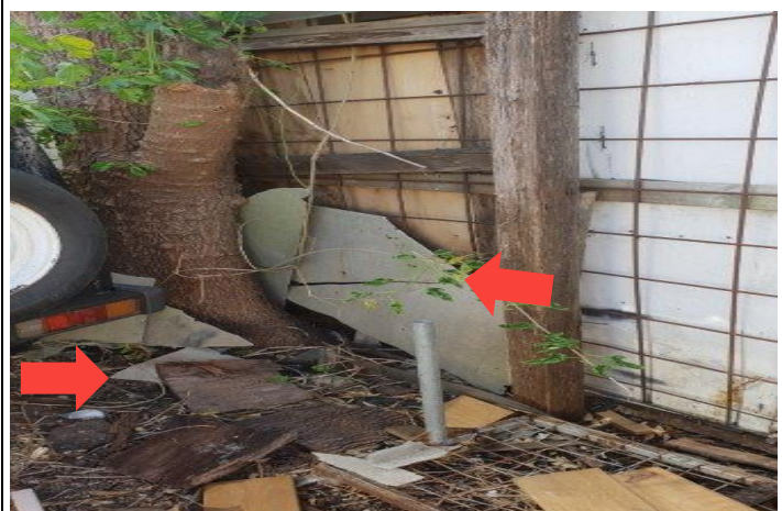
Photo 10: 134 Parramatta Road, southern timber wall frame, asbestos-containing fibre cement sheeting observed.
