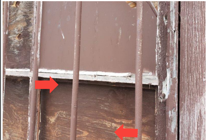
Photo 12: 38 Good Street, Western elevation, asbestos-containing fibre cement infill panel to window
