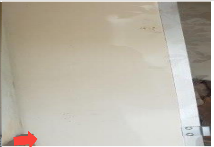
Photo 14: 38 Good Street, Western Elevation, Female Toilets partition walls asbestos-containing fibre cement Sheetting.
