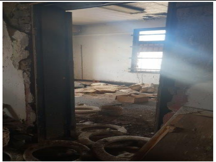
Photo 32: 38 Good Street, first floor, eastern room, walls, lead containing grey paint (WSP-104456).
