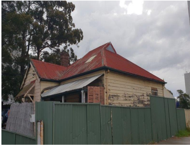
Photo 19: 59 Cowper Street, Dwelling – Exterior, Roof gutters, lead containing green paint (WSP-104431).
