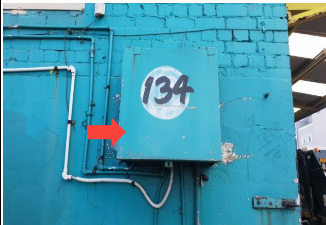
Photo 9: 134 Parramatta Road, north western corner to lot, asbestos-containing electrical distribution board.
