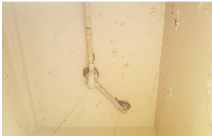
Photo 34: 38 Good Street, first floor, Western elevation, exterior toilet walls, lead containing white paint (WSP-104461).
